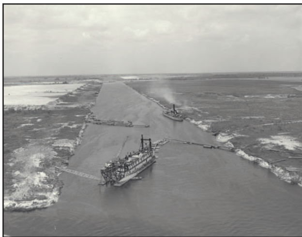
Dredging of the Kissimmee River into a 30 foot deep straightaway called the C-38 canal as part of Central and South Florida Project
